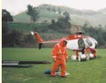
A Powerco Energy Services crew prepares a helicopter for an aerial line-hanging mission
