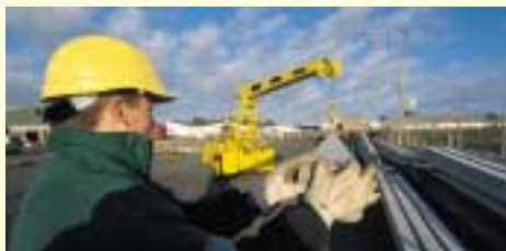
A Powerco Energy Services line mechanic works with a crane operator to remove power poles from a depot
