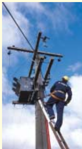
A Powerco Energy Services line mechanic replaces fuses on an 11kV line
