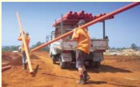
Powerco Energy Services Australia crew carry out installation of an underground conduit for electric cabling in a new subdivision in south Queensland
